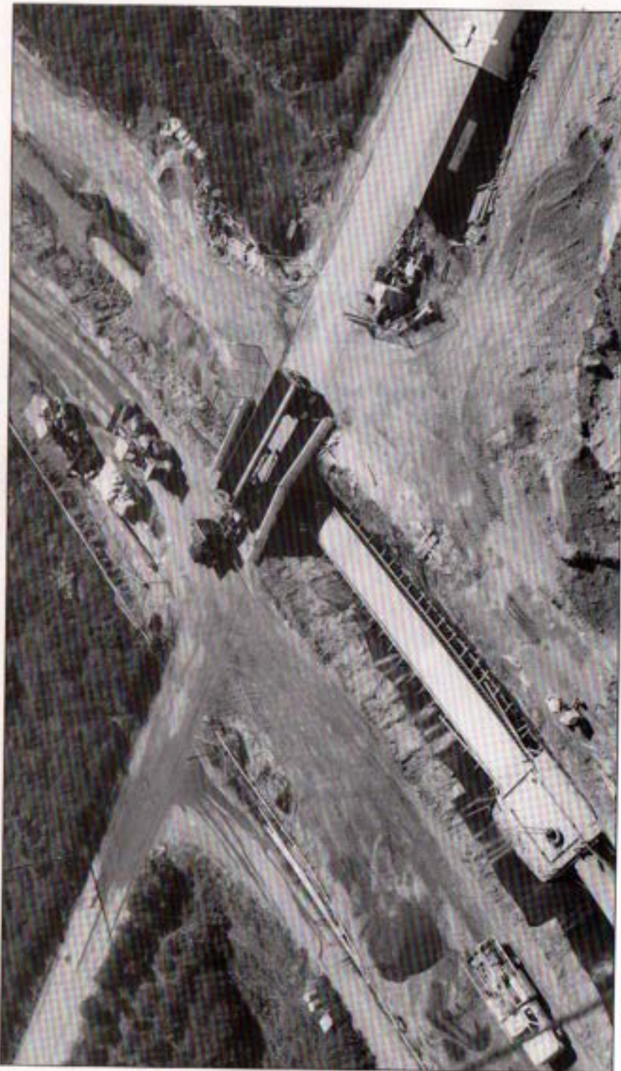
Aerial View of the 72-inch North County Distribution Pipeline and Encasement at the Twin Oaks Valley Road Crossing.
