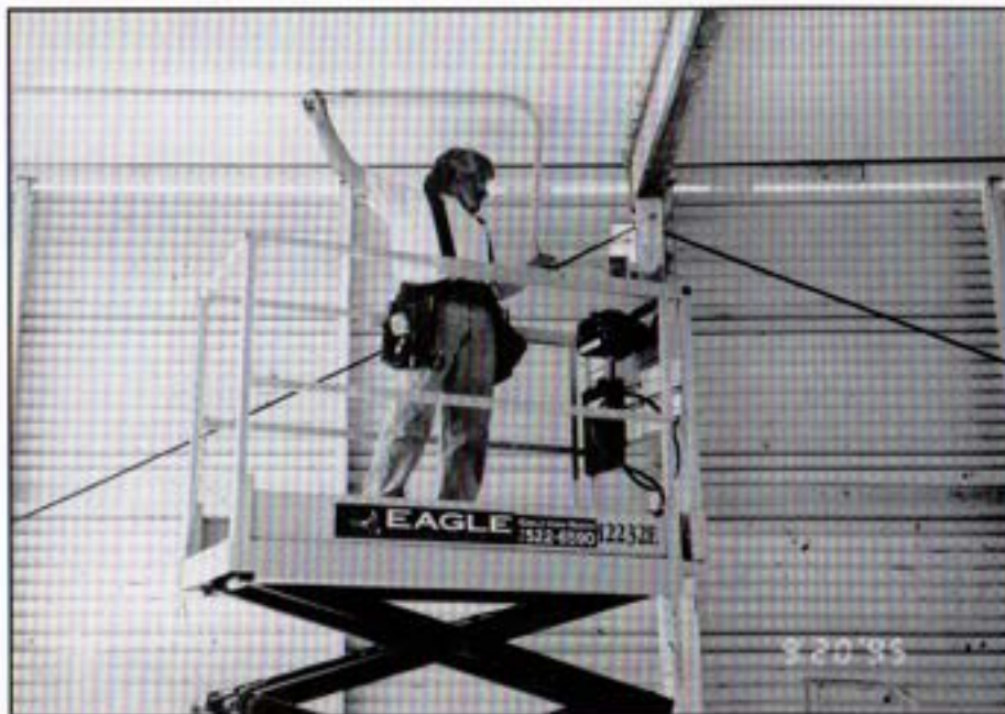
System Technician Gene Bencivenga installs conduit for yard security lighting at the Escondido Operations Center.
