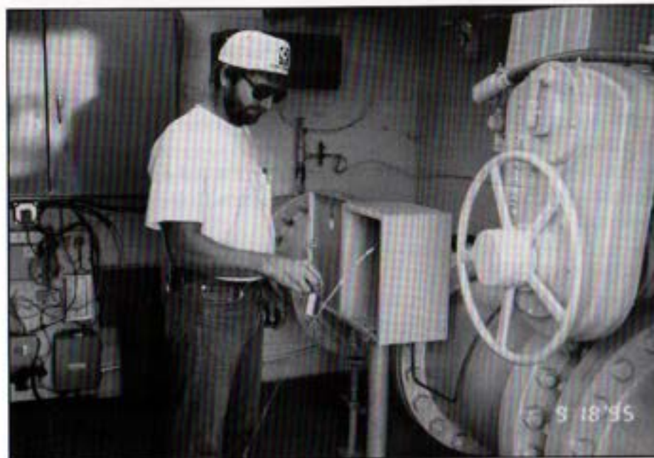
Systems Operator, Greg Nelson takes a water sample for bacteriological testing at the Oceanside #3 Flow Control Facility.
