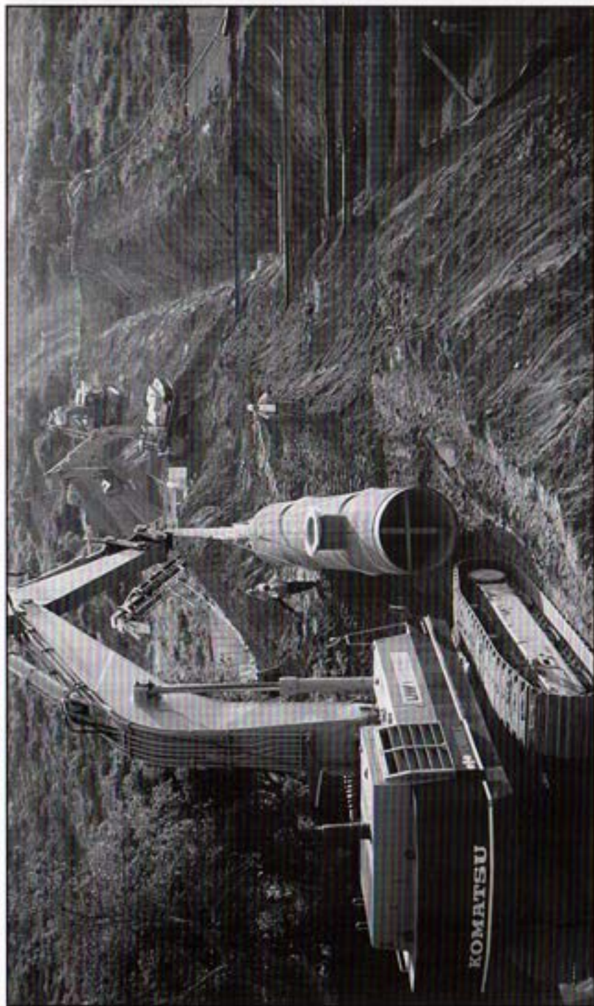
Excavation setting to place the first 40-foot long section of 72-inch diameter pipe for the North County Distribution Pipeline.
