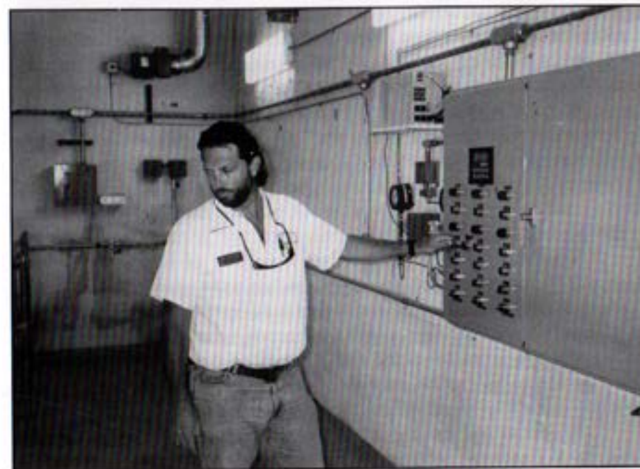
Systems Operator, Joe Wegand makes adjustments to modulating valves in the Diversion Structure.
