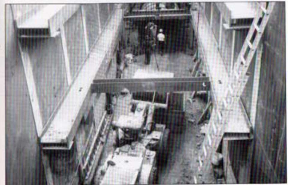
Excavator equipment constructing the tunnel below the city of San Diego's 66-inch PCCP Miramar Pipeline.
