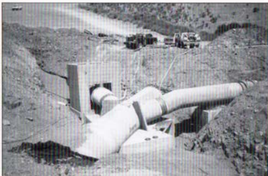
Connection of the Scripps Ranch Pipeline to Pipeline 3. The work was designed to accommodate connections to future pipelines.
