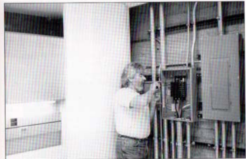
Systems Technician Gene Bencivenga installs a new panel board as part of the Supervisory Control and Data Acquisition (SCADA) system.
