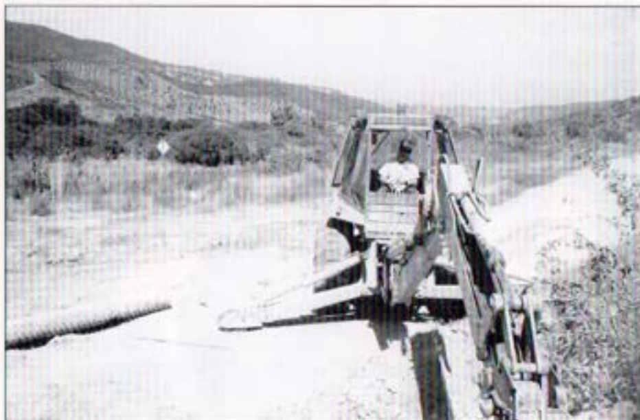
Senior Maintenance Specialist Lewis Russo installs a culvert to control erosion damage to access road.
