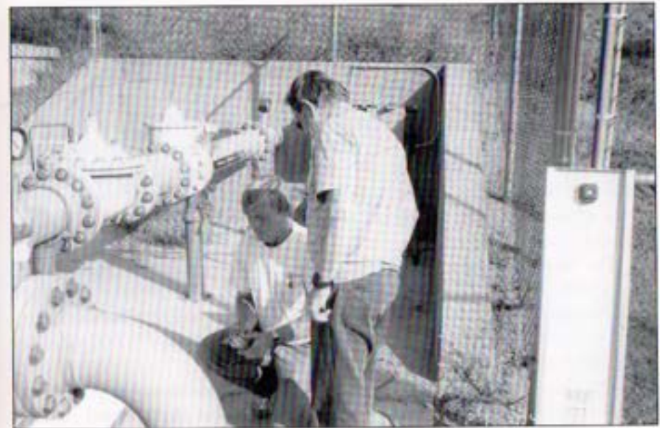
Senior Systems Technician Greg Tucker and Systems Technician Bob Catalano layout a solar power panel at Rainbow #13 Flow Control Facility.
