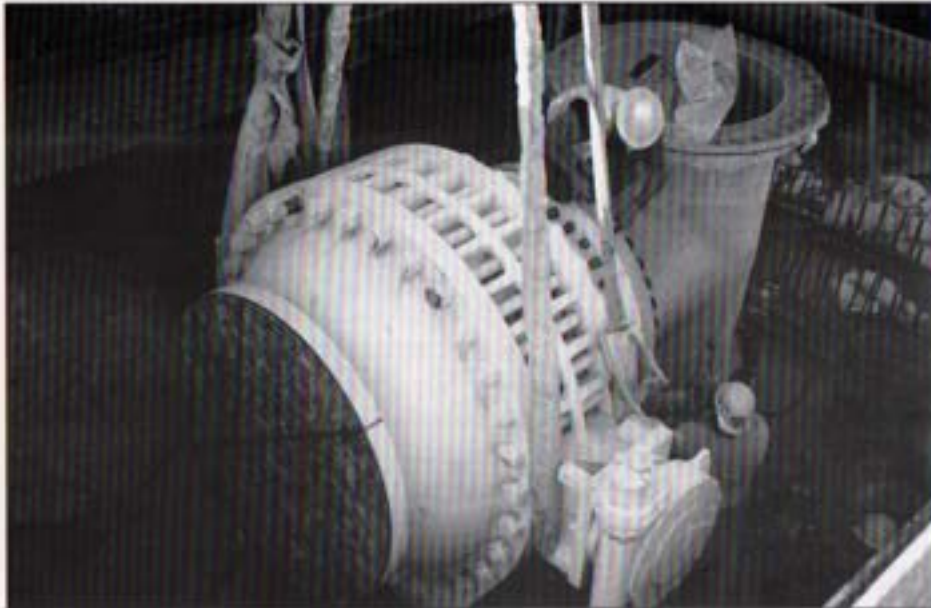
The La Mesa/Lemon Grove Pipeline included installation of a 48-inch ball valve to serve the city of San Diego and Helix Water District.
