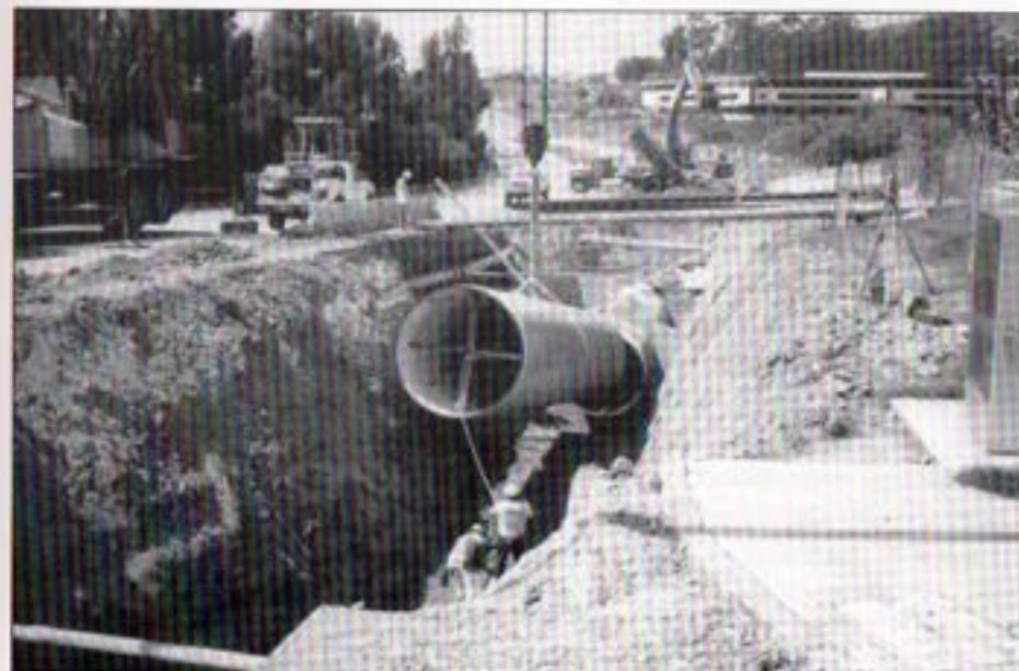
Installation of 96-inch diameter pipeline along Scripps Ranch Boulevard. Trench backfilling operations are proceeding in the background.
