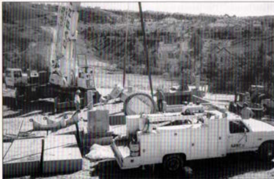
Installation of a 60-inch butterfly valve south of State Route 52. The valve is used to isolate the Scripps Ranch Pipeline at its connection with Pipeline 4.
