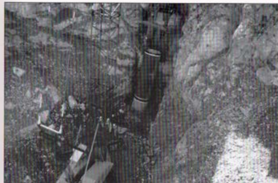
Lower Otay Pipeline installation progressing up the south side of the Sweetwater River embankment.
