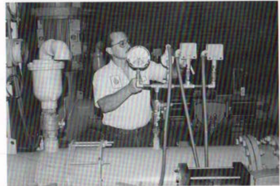
Senior Systems operator Ed Hartzler makes adjustments to instrumentation at the Escondido Pump Station.
