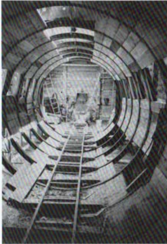
Soft ground tunnel under San Miguel Avenue. Looking through the tunnel at the entrance portal.
