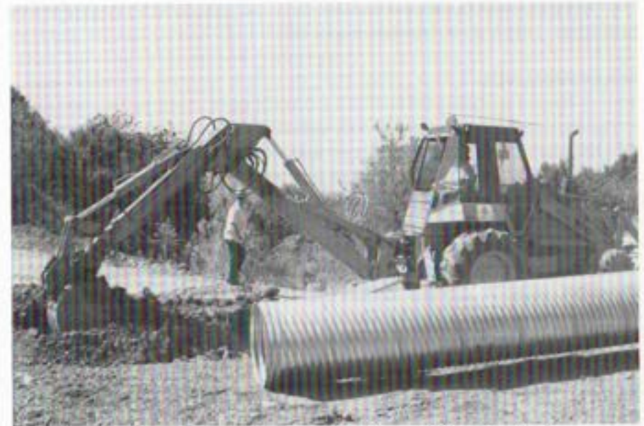
Equipment operator crew installing a 30" galvanized culvert on right of way access road.
