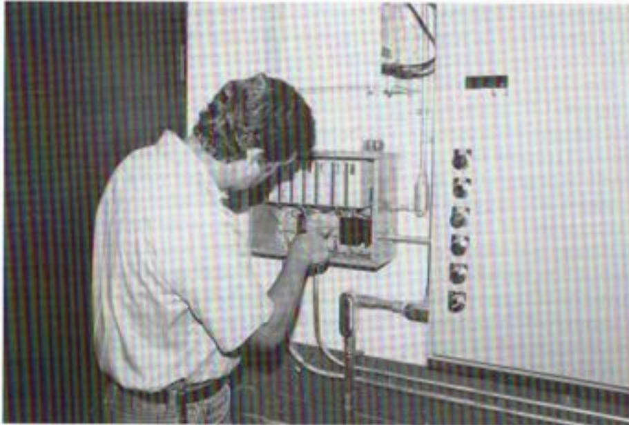
Chet Kalinowska, System Technician, performing final hookups on a new programmable logic controller at Rincon #1 flow control facility.
