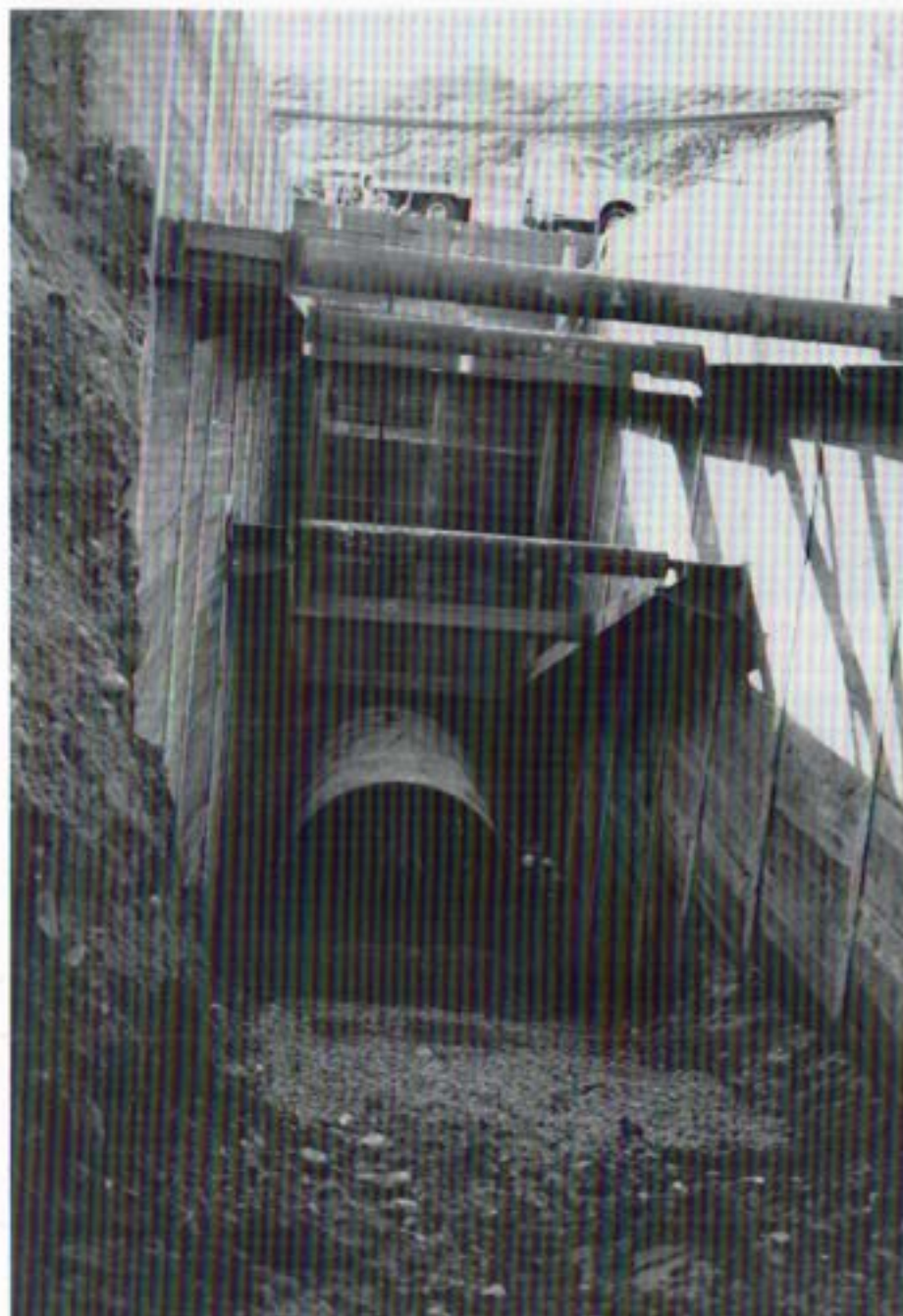
Tunneling operations for the La Mesa-Lemon Grove Pipeline. This 96-inch diameter tunnel is located under Jackson Drive.
