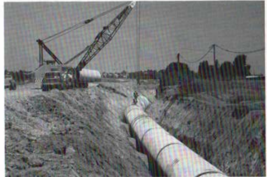
Installation of the 108-inch diameter San Marcos Pipeline through environmentally sensitive area.
