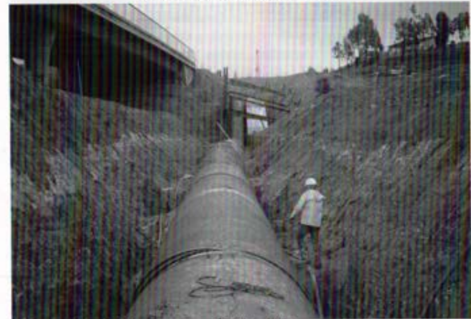
Partially backfilled section of 108-inch diameter pipeline across the future extension of State Route 56. The work was part of the Rancho Penasquitos Pipeline project.
