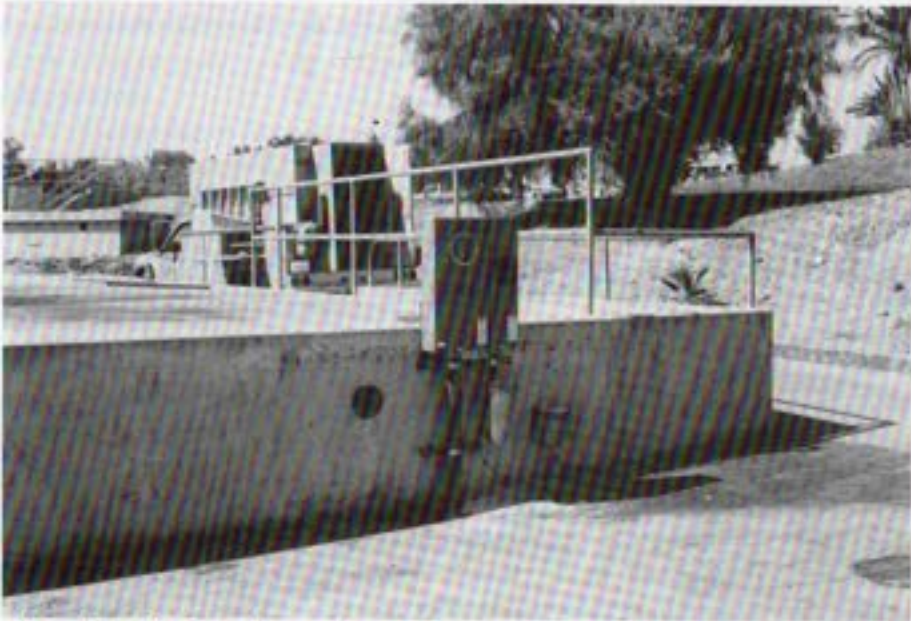
New electrical services such as this are installed at various flow control facilities as part of the upgrade program to modernize the systems within the station.
