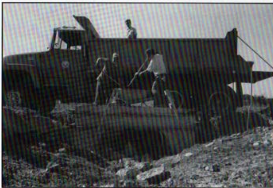
Maintenance personnel Steve Carpenter, Al Earnest and Bruce Rudolph build a headwall at the Olivenhain 3 Service Connection.
