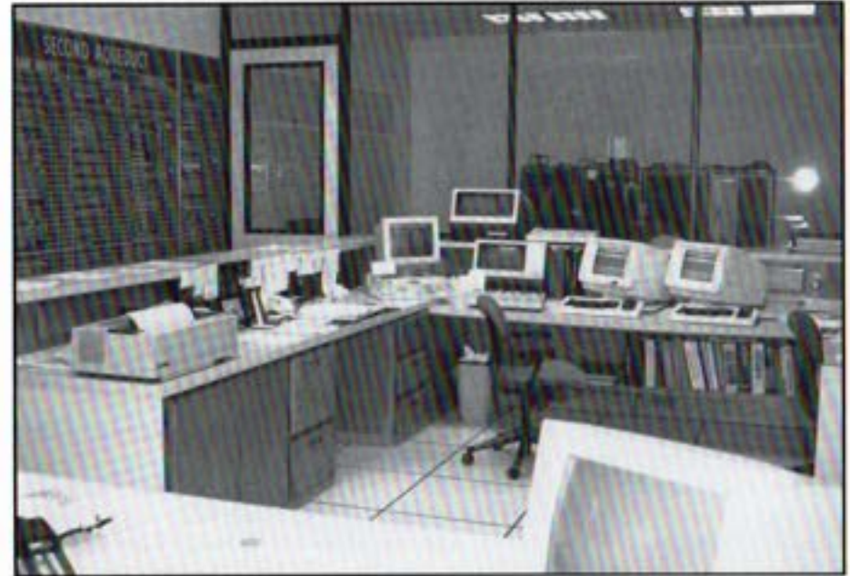
The Authority's computerized control room in Escondido. The control room is operated seven days a week to monitor and control flows to all member agencies.
