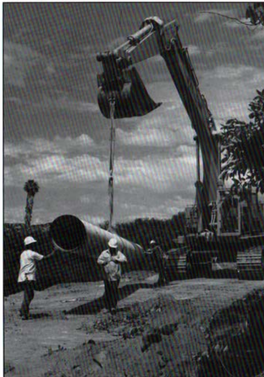
A 30-inch pipeline from the Crossover Pipeline to the pump station is constructed as part of the Escondido raw water pump station and modifications to the First San Diego Aqueduct.
