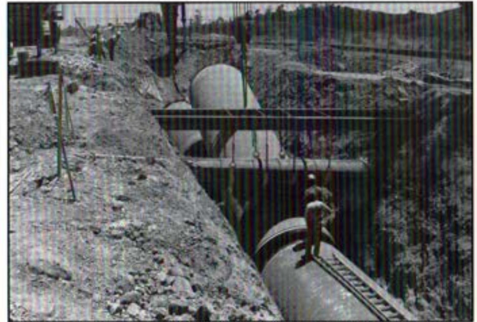
Construction foreman carefully guides a 40-foot section of 108-inch diameter pipeline into position. Directly above the pipelaying a fully supported Vallecitos Water District 30-inch waterline remains in use.
