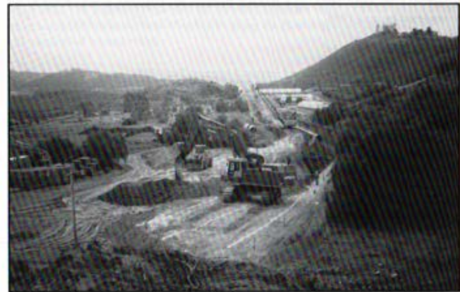
Excavation continues along the pipeline alignment. An excavator is shown digging trench in the foreground while a crane continues pipelaying activity in the background.
