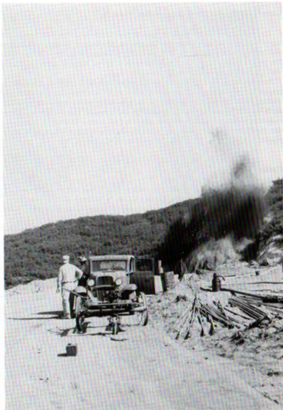
Blast set off to open cut at North Portal Lilac Tunnel - 1947 San Diego County Water Authority - Photograph Collection
