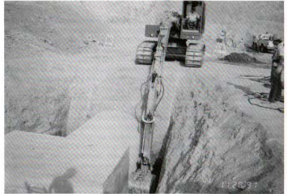
Lewis Russo (on rig) and Steve Carpenter operate the Authority's Operations and Maintenance new crawler backhoe to excavate trench for the Highway 56 encasement project for the 4th barrel of the Second Aqueduct.
