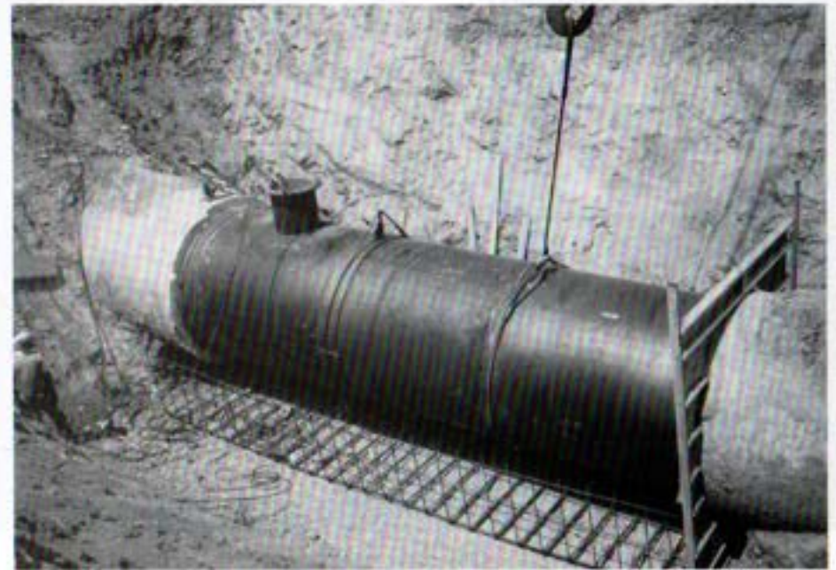
The steel replacement pipe for the repair of the 84-inch Pomerado Pipeline completely installed.
