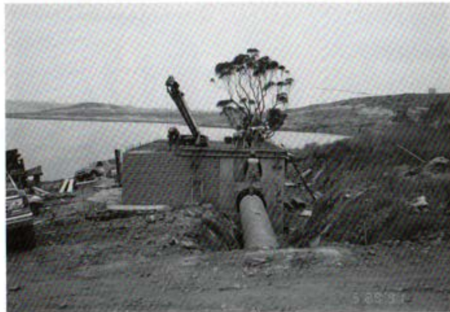
Construction of flow control facility for delivery of water to Sweetwater Reservoir
