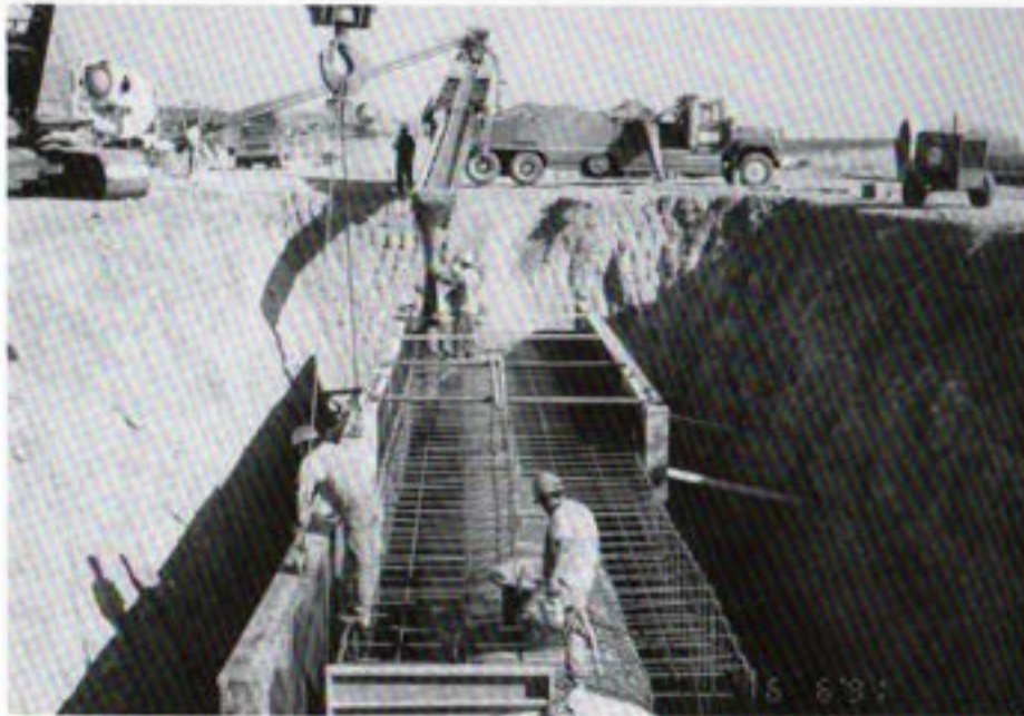
Forming reinforced concrete encasement for repairs of the 84-inch Pomerado Pipeline, June 1991
