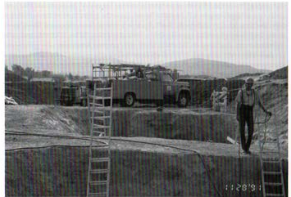
Operator Will Kane acts as safety lookout while Authority crews work in trench for the Highway 56 encasement project on the 4th barrel of the 2nd Aqueduct.
