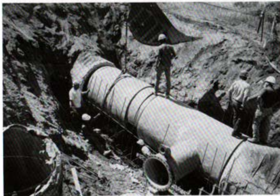
Completed 30-inch connection at Crossover Pipeline for Escondido Raw Water Pump Station
