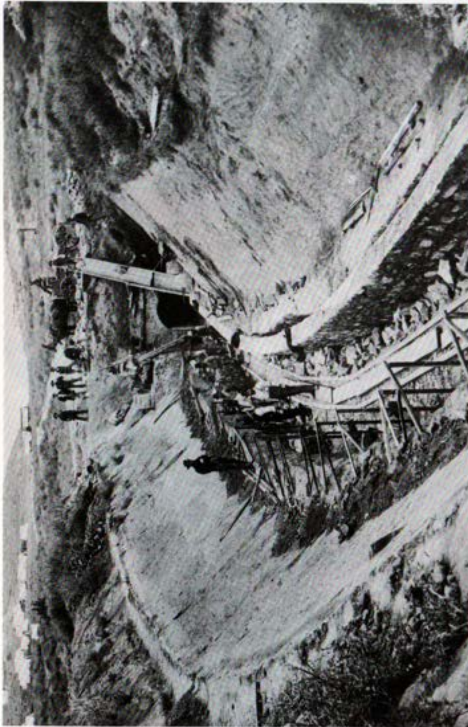
San Diego Cuyamaca tunnel and camp for flume—Circa 1887 San Diego Historical Society—Photograph Collection
