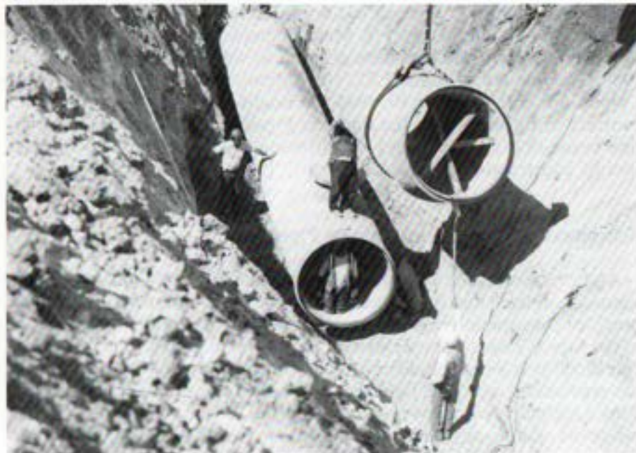
RAMONA PIPELINE PROJECT 1988-89 Laying over 8 miles of 54-inch to 36-inch diameter pipeline to serve the City of San Diego (Rancho Bernardo area), the service areas of the Ramona MWD and Olivenhain MWD
