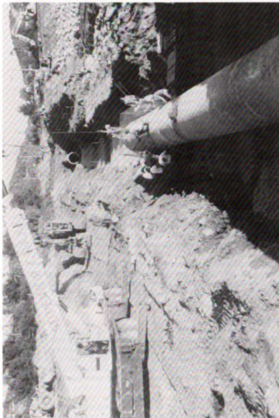
Laying 262 feet of the 66-inch diameter crossover pipeline to accommodate improved flood control channel in the City of Escondido -- 1988
