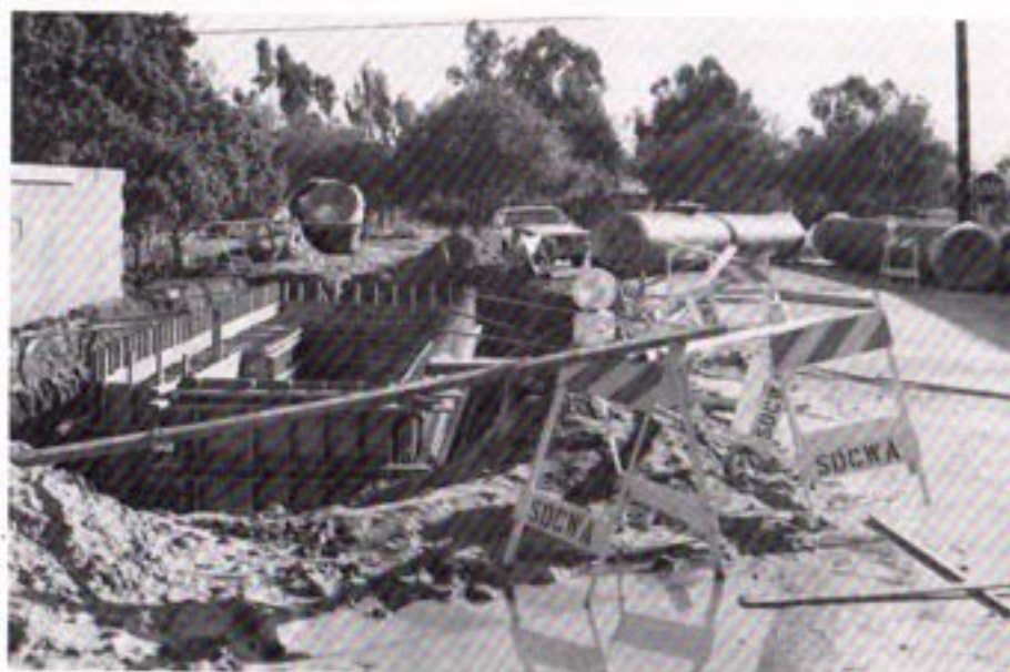
New San Diego Service Connection No. 13 at Gillespie Drive and Jamacha Blvd. during construction this year. Note size of pipeline that this connection will serve.
