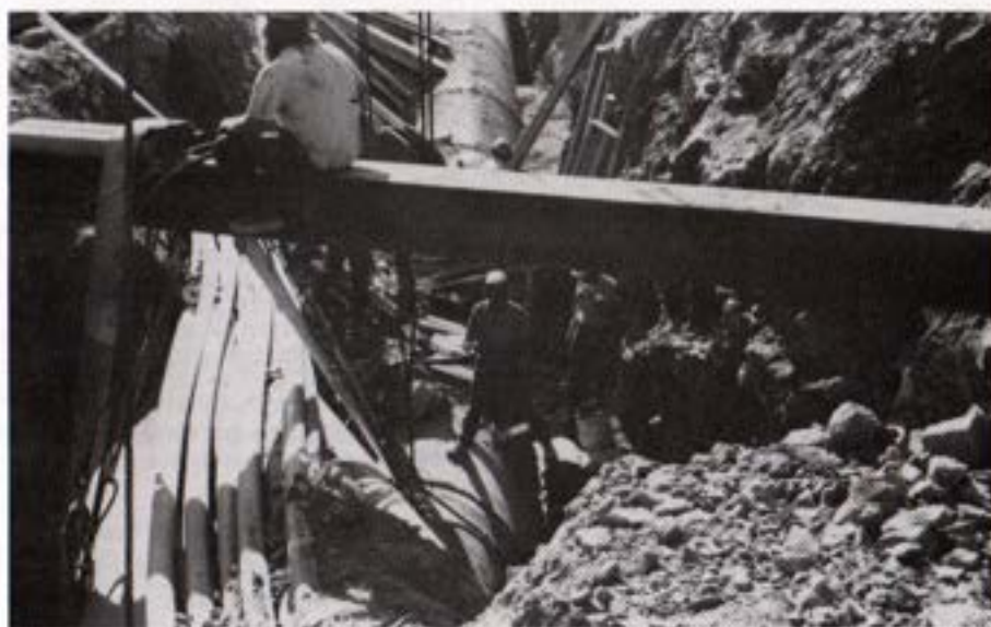
Crossing below the City of San Diego's 66-inch water line that supplies the northern half of the city. The solid rock beneath the city pipeline had to be broken hydraulically.
