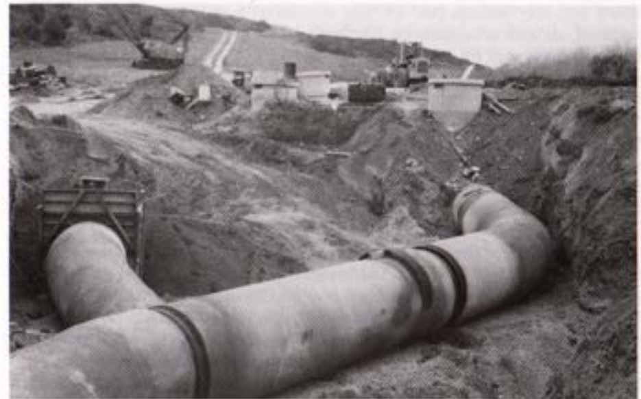
Interconnection of Pipelines 3, 4 and 4A (left to right) nearly completed. Connection 4A-4 backfilled. Connection 3-4A ready for closure. Looking east.
