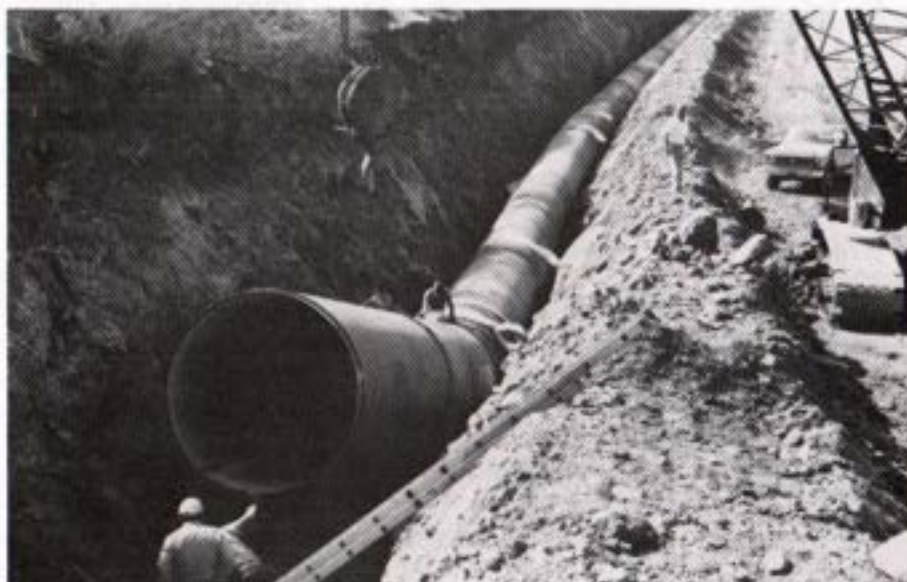
Laying 40-foot lengths of Pipeline 4A. This is 72-inch diameter mortar lined and coated steel pipe with each joint completely welded in the field.
