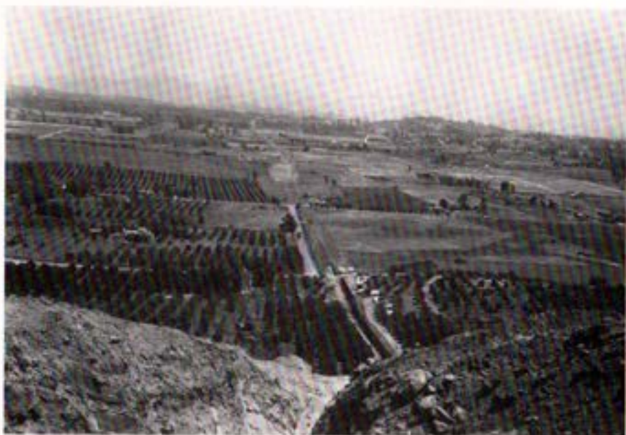
A view of the First Aqueduct under construction in 1946 and looking south through the City of Escondido.
