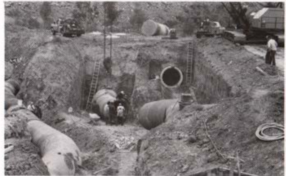
Interconnection of Pipelines 4A, 4 and 3(left to right). 4A-4 ready for closure; 4-3 laying the pipe; 3-4A must wait for backfill of other connections. Looking west.
