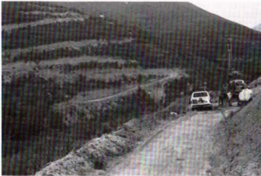
Core drilling for determination of the depth and strength of foundation rock at the north abatement and looking across at the south abatement.
