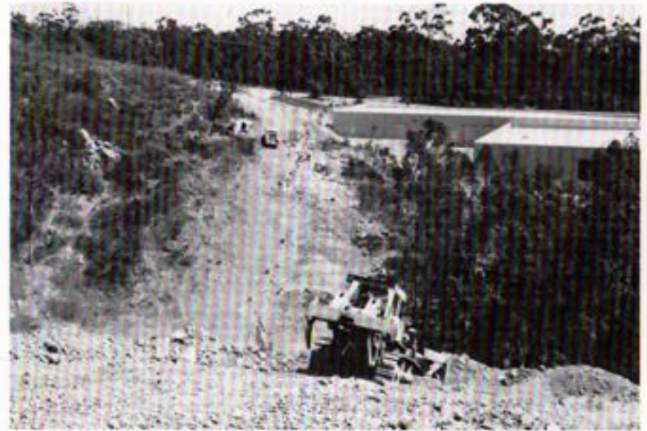
Another view of Pipeline 4A showing the pioneering, drilling and blasting near a highly developed commercial area.
