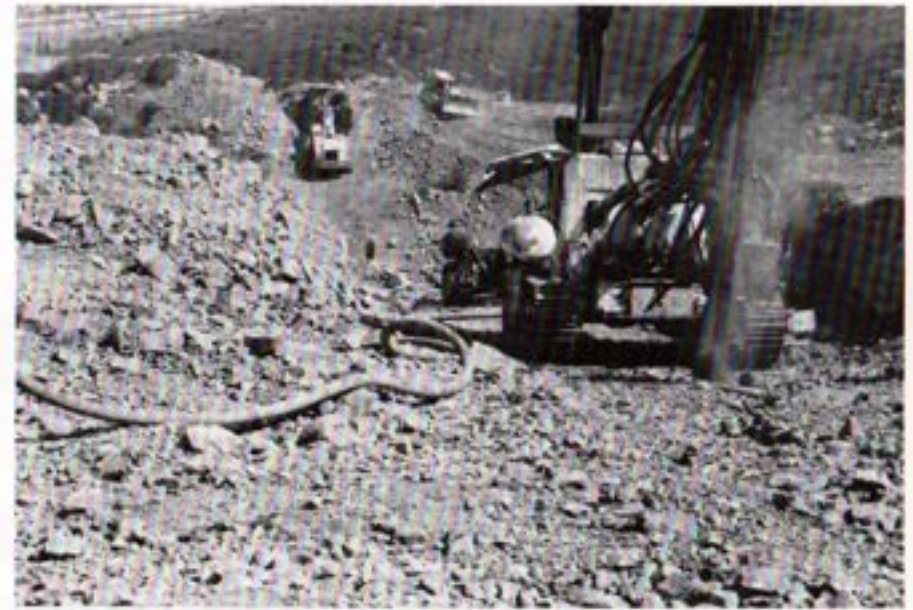
Pipeline 4A required extensive rock drilling and blasting prior to excavation of the trench.
