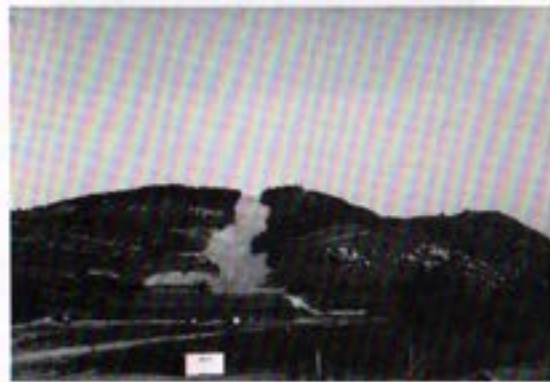
View of north slope of San Luis Rey Valley after finish backfill.
