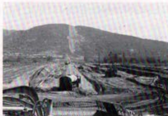
Scrapers were used to excavate trench across the San Luis Rey River and stockpile material on upstream side of the trench. A very extensive dewatering system was required.
