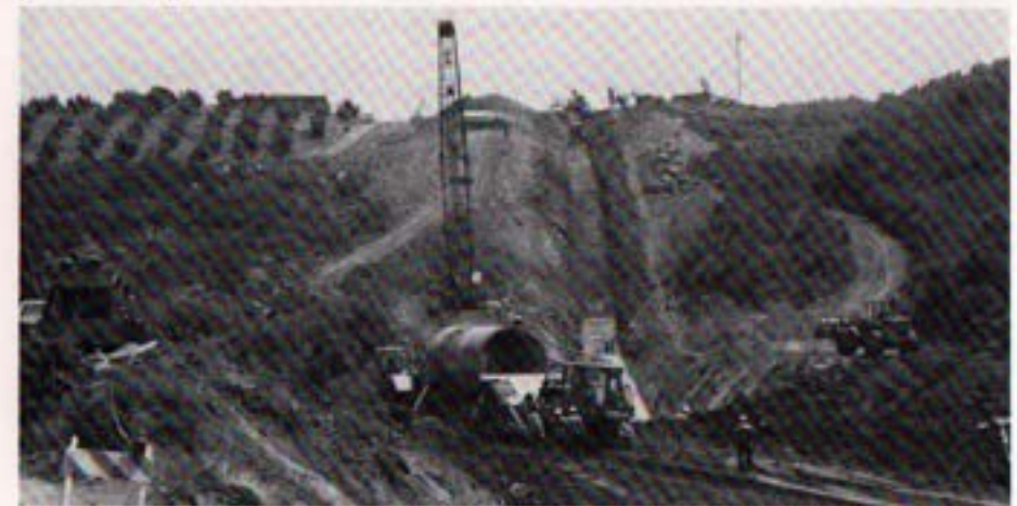
Specially-constructed transporter hauls pipe from storage yard to laying site where crane places pipe section directly into the trench.
