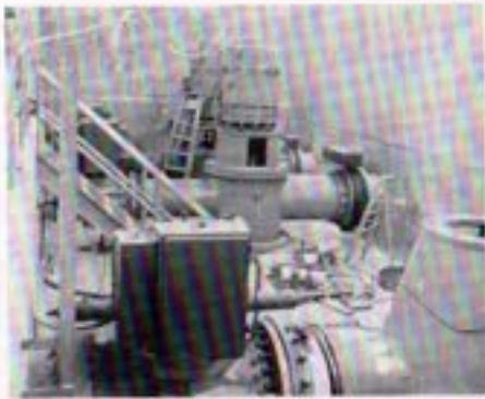
Interior view of pumping plant showing two pumps nearing completion. Total of all pumps installed will be 2,800 horsepower when completed. Station was about 75% complete at end of fiscal year.
