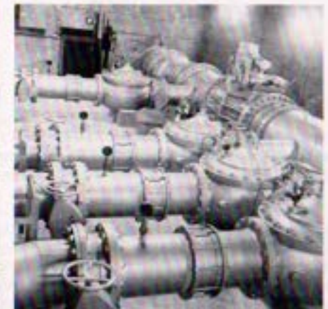
Pipeline 4 Extension to Alvarado Treatment Plant, completed in January 1978, terminates in pressure reducing system in San Diego No. 12 Service Connection, which was constructed under the pipeline contract.
