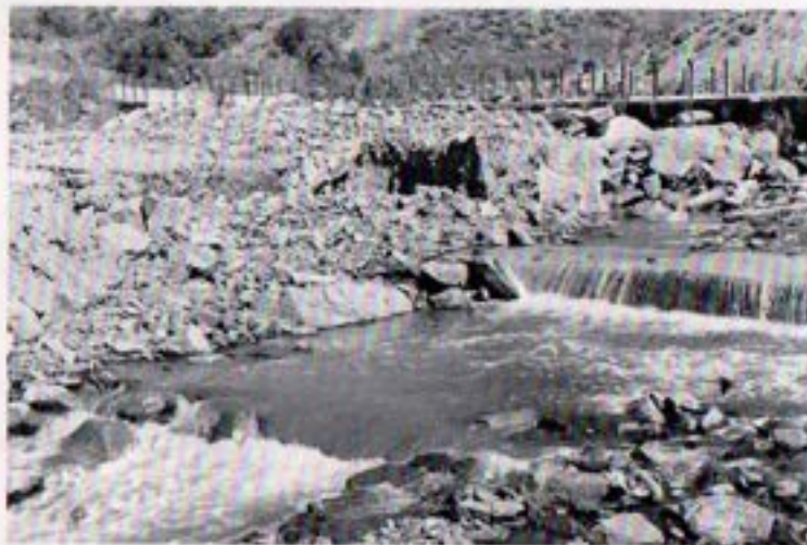
Heavy rains during February and March 1978 caused severe erosion in several of the major streams in San Diego County. San Diego River in Mission Gorge is pictured with Pipeline 3 encasement exposed. Pipeline 4, constructed during 1977, was also exposed at this river crossing.
