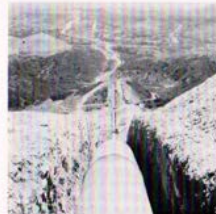
Pipeline 4 construction in rugged area north of Mission Gorge affords panoramic view of developed area of northeast San Diego. Jackson Drive, alignment of pipeline in upper left background.
