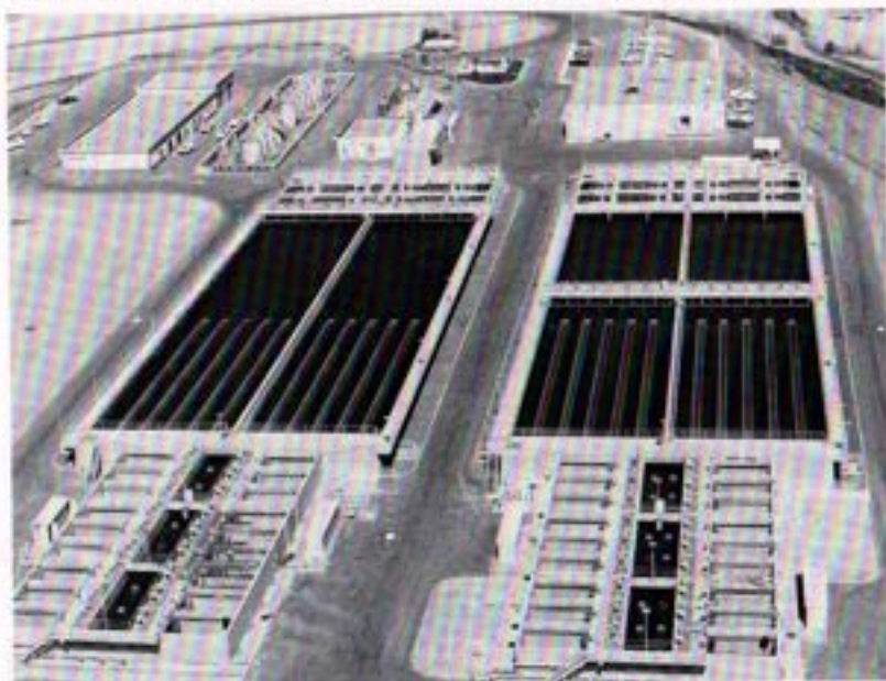
Robert A. Skinner Treatment Plant nears completion. Primary features are main control building (upper right), mixing basins and settling basins (center right and left), and filters (bottom right and left). In background are shops (far left) and chemical storage tank area. Center background is plant control and electrical equipment building. (Photo courtesy MWD)
