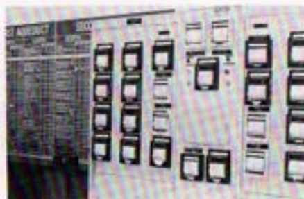
Flow indicators with telemeter signal from service connection to Escondido Operations Center. Nearly one-half of the service connections are now controlled by this means.
