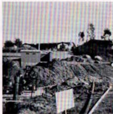
Poway No. 3 Service Connection at Stoneridge Golf Course. Structure replaces air release valve enclosure on Pipeline No. 2. Piping in foreground are customer installation. Service connection structure construction by SDCWA forces.
