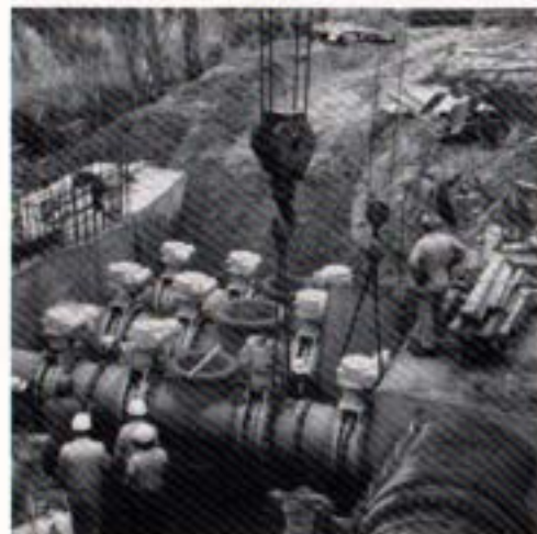
Valves at Interconnection near Miramar Dam. Specification 223
