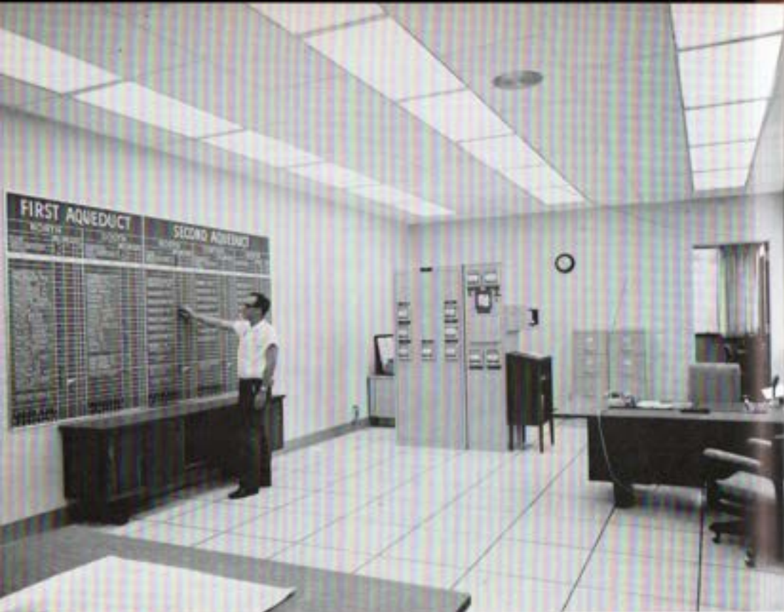
Control Room, Fred A. Heilbron Operations Center
