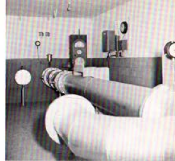
Interior View of Yuima Service Connection
