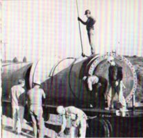
66 inch Pipe Special for Cross-Connection
