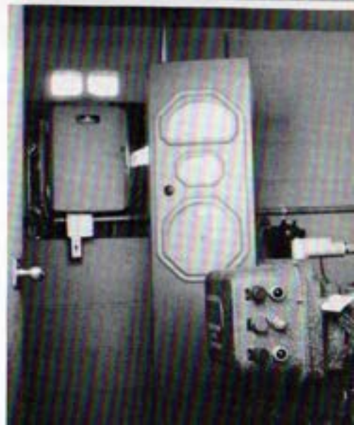
Maintenance and Operation Equipment
