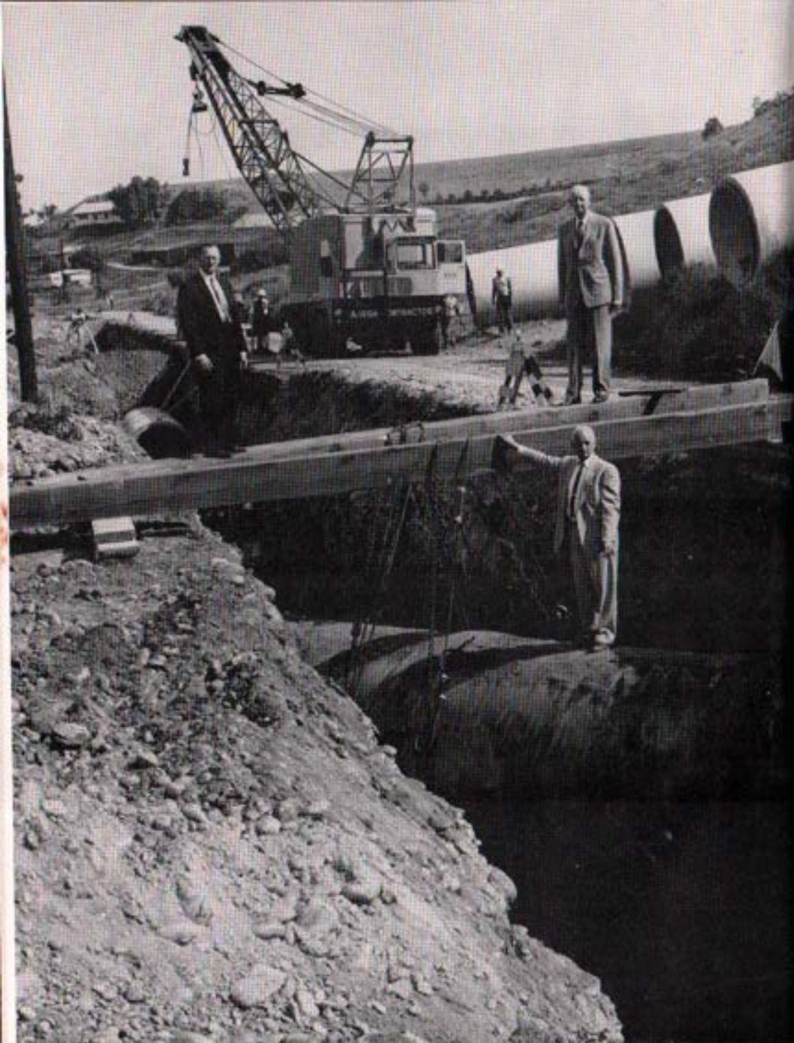
Messrs. P. Beermann, F. Heilbron and R. Holmgren Inspecting Second Aqueduct Crossing Under City of San Diego's El Monte Pipeline at Baltimore Drive in La Mesa
