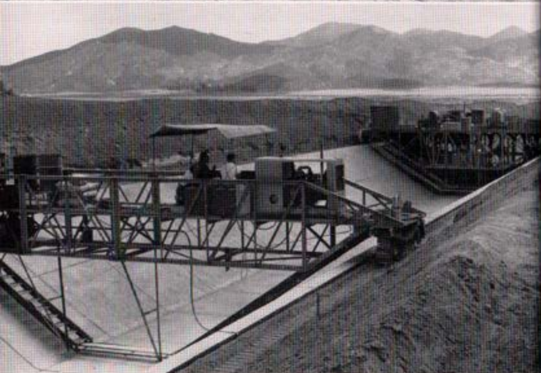
Placing Concrete Lining on Metropolitan Water District Canal Section of Second Aqueduct
