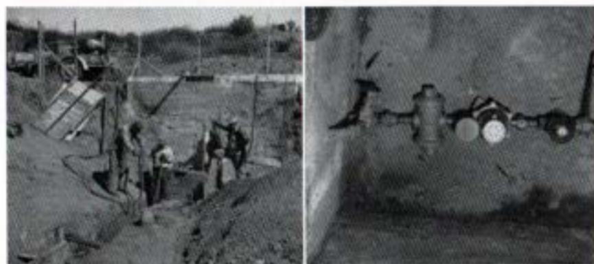
Determination of Leakage into Red Mountain and Oat Hills Tunnels, and Provision for Discharging Leakage from Aqueduct
