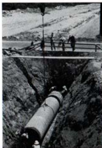
Placing 48-inch Steel Pipe Adjacent to State Highway No. 76, Near San Luis Rey River.
