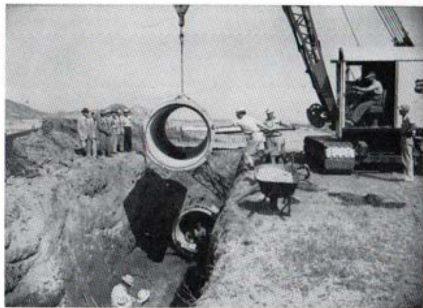
Laying First Pipe of Second Barrel of San Diego Aqueduct near Winchester
