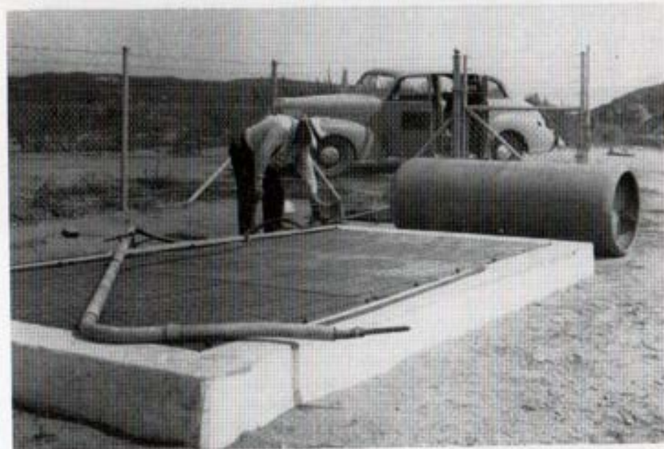
Equipment used to inject Chlorine into Aqueduct at Bifurcation Structure North end of Lilac Tunnel
