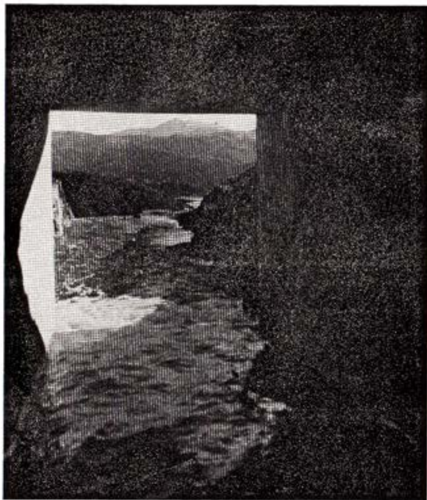
First flow of water from San Diego Aqueduct at south portal of San Vicente Tunnel into San Vicente Reservoir, November 26, 1947.
