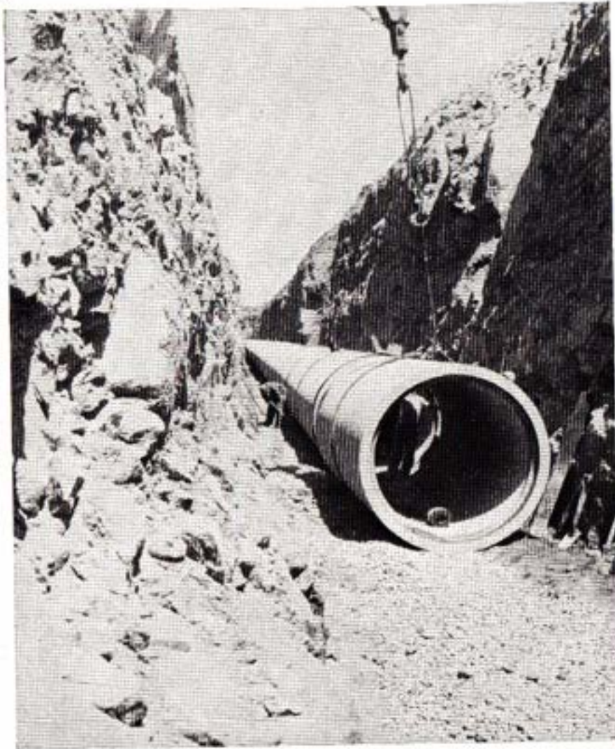
Placing 72" pipe at North approach to Poway Tunnel (Station 214), San Diego Aqueduct.
