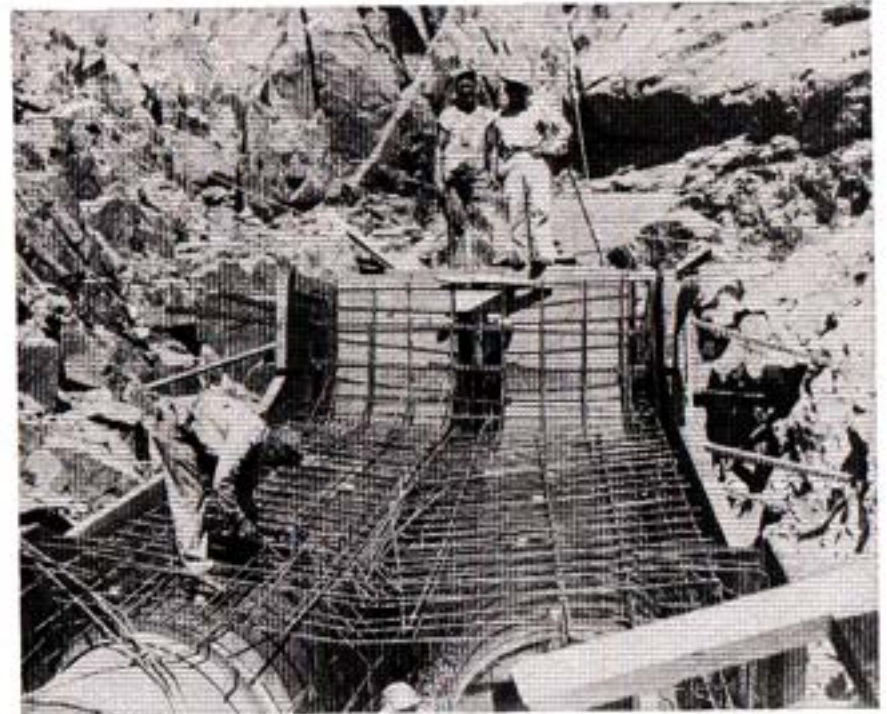
Placing reinforcing steel for concrete bifurcation structure at North portal of San Vicente Tunnel.
