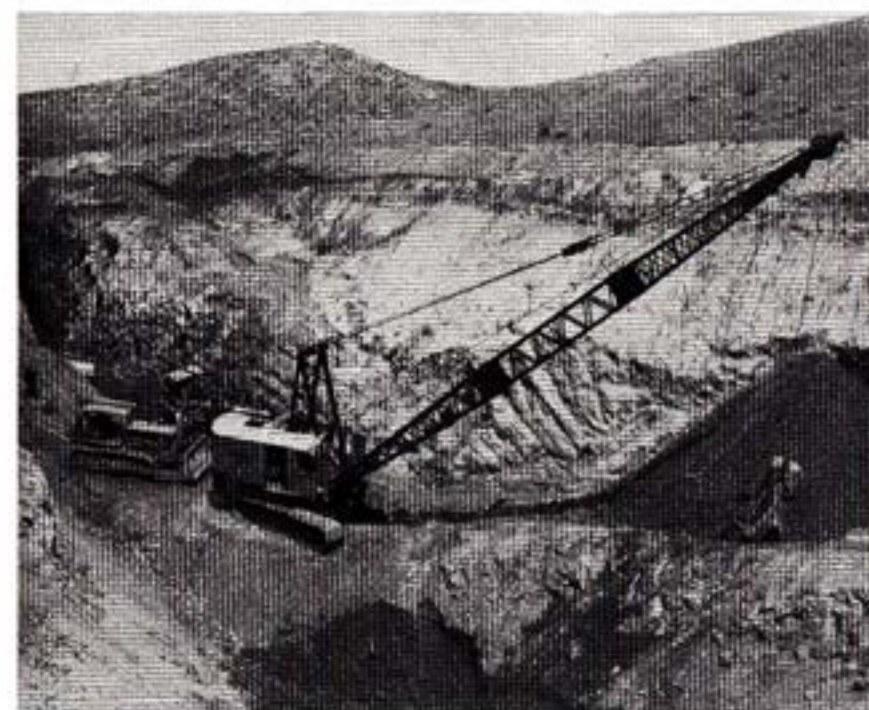
Excavating for 72" pipe, North approach to Poway Tunnel (Station 212), San Diego Aqueduct
