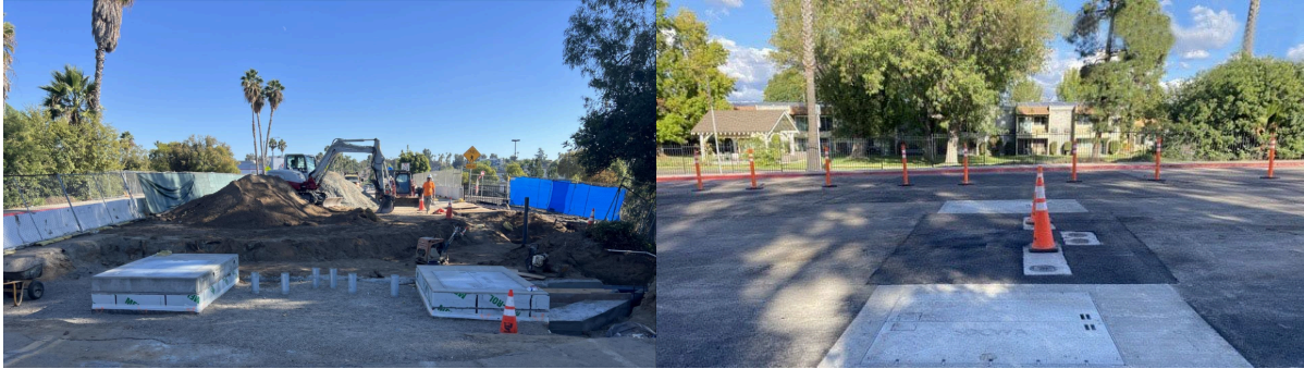
Left: Two newly installed access vaults along Harding St. Right: Newly paved road following structure upgrades, with traffic-safe plating.
