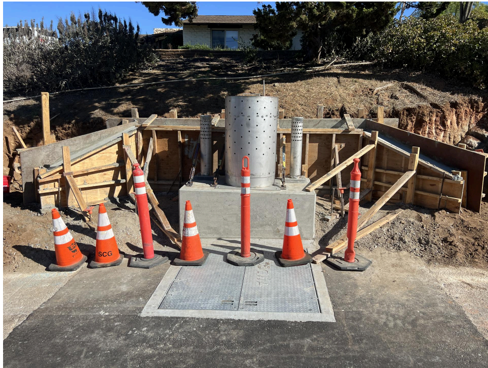
Restoration begins on an upgraded pipeline structure, preparing the site for upcoming inspections.
