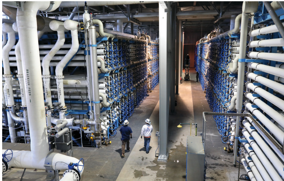
The Carlsbad Desalination Plant produces up to 54 million gallons per day of locally controlled water for San Diego County.
