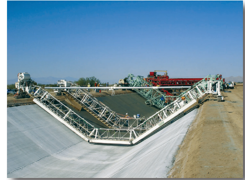
The Water Authority has secured additional Colorado River supplies through canal-lining projects.
