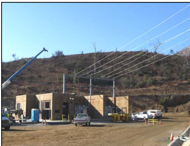
The new light tan-colored varnish is on the exterior of the pump station.
