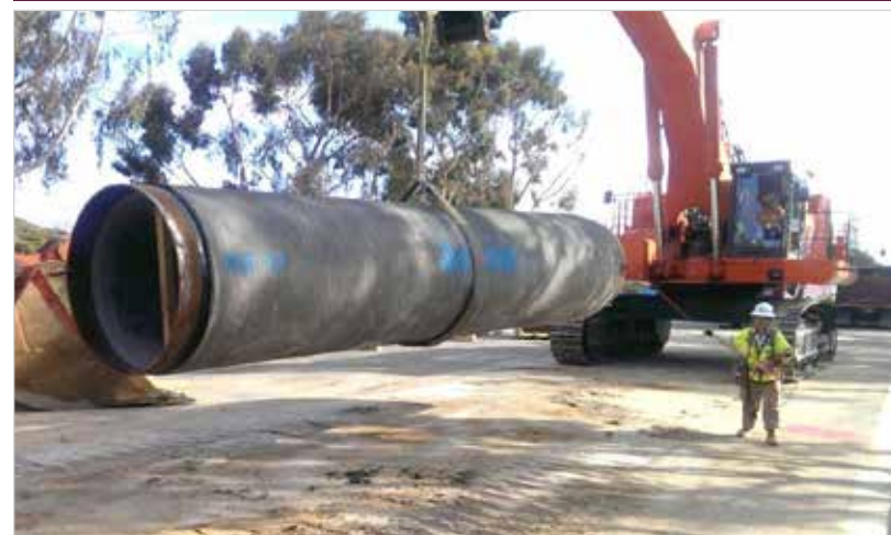
Work crews install a section of 54-inch steel pipe connecting the Lewis Carlsbad Desalination Plant to the Water Authority's aqueduct system.
