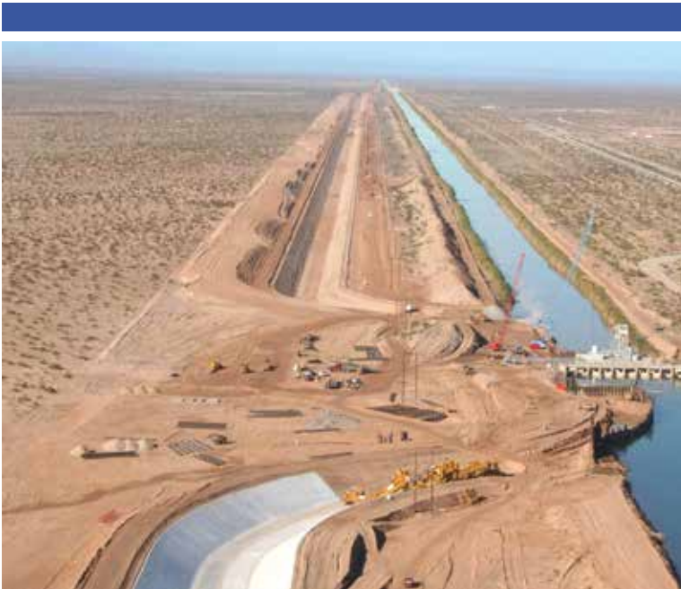
As a result of the Quantification Settlement Agreement, the lining of the All-American Canal contributes to San Diego's imported water supply.
