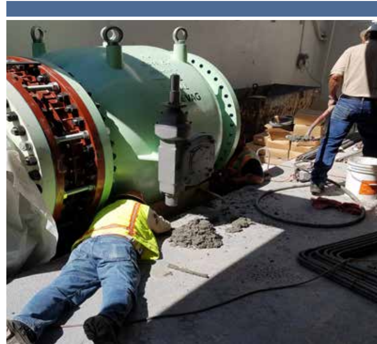
Crews repair equipment at one of the Water Authority’s flow control facilities.
