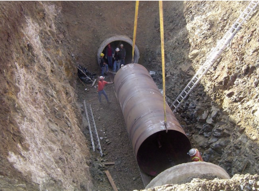
A steel liner section being lowered into the portal to be inserted into the existing pipe.
