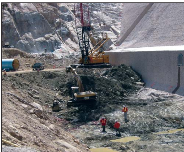
The dam raise will have a new foundation up to 25 feet deep and extending 75 feet out from the toe of the existing dam (upper right).
