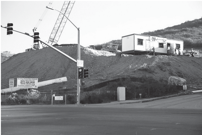
This site will be the home for a San Vicente Pipeline shaft and a pressure control and hydroelectric facility.
