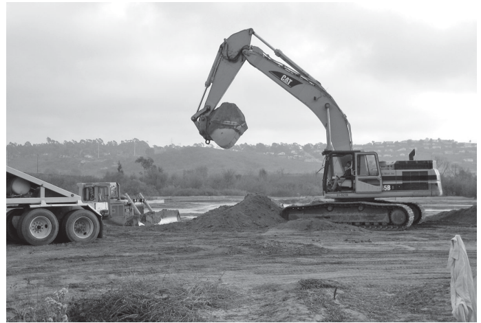
Approximately 24,000 cubic yards of materials were removed to create new wetland habitat.
